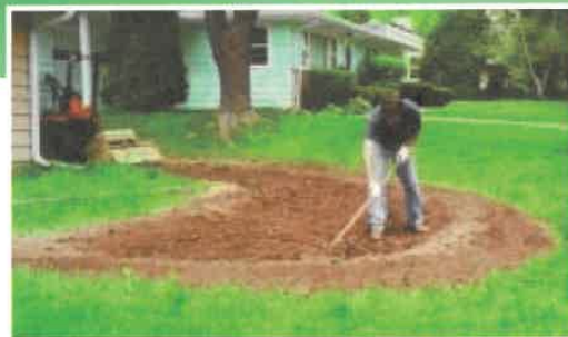
On a gentle slope, soil from digging out the garden can be used to create the berm.
